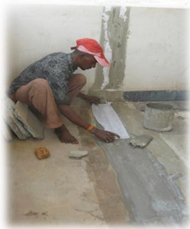
Electric panels installation and waterproofing of the hospital walls thanks to the financing and to the technical specifications of partners specialized in the domain.
